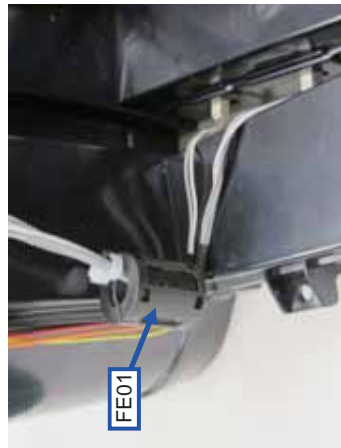
(1)-7 Wiring after closing the lid of the PANEL DUCT - 3 Put FE01 attached to CNISS and CNOSS as shown in the picture.
